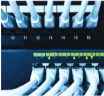
Hubs and Switches
