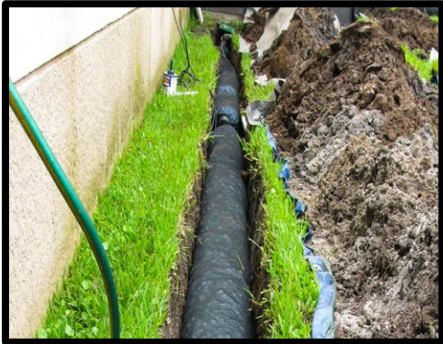
Drain carrying dirty water
