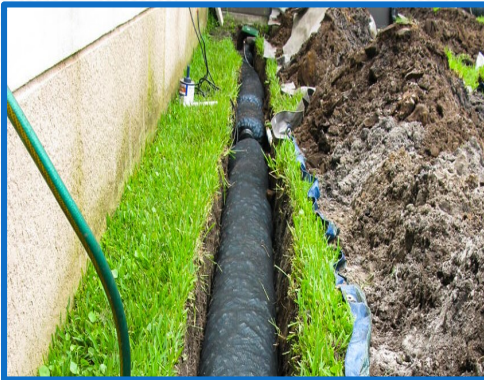
Drain carrying dirty water
